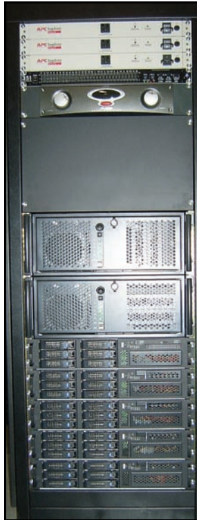
Figure 7-4. Student training station computer rack.
